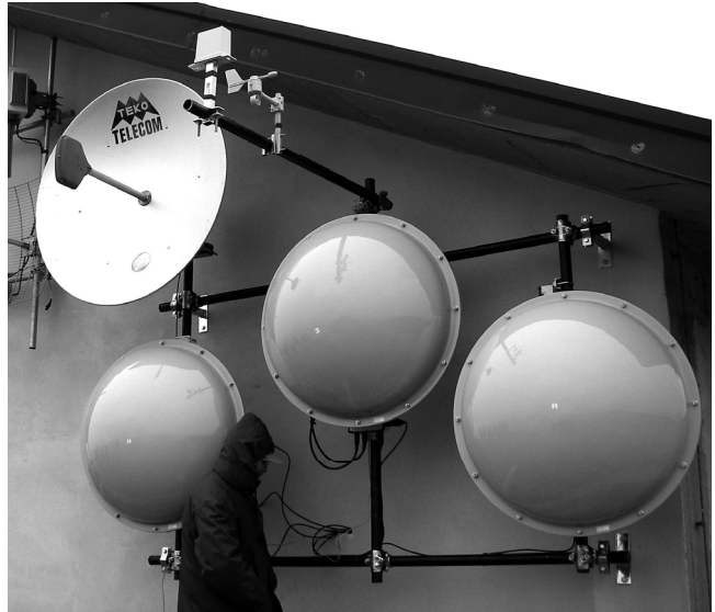
Figure 5: Physical installation at Monte Cesen.
